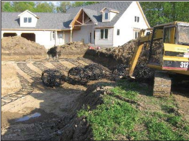
The geothermal ground loop is laid in front of the Henig home on Zeeb Road in May 2008. The system transfers heat like a large radiator in the soil.
